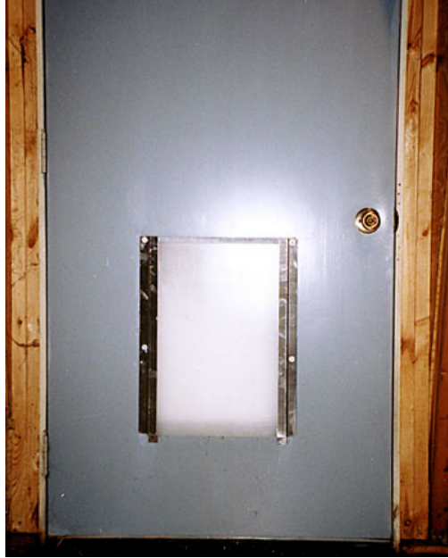
An installed closure on metal door Photo 2
